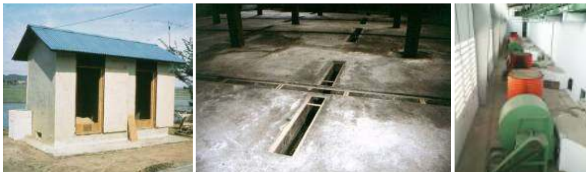
Figure 23: Korean low-temperature in-bin drying and storage system (IBDS) at farm level (left), aeration ducts in a large storage system (center), and blowers and heaters for an in store drying system with 4 batches (right).
